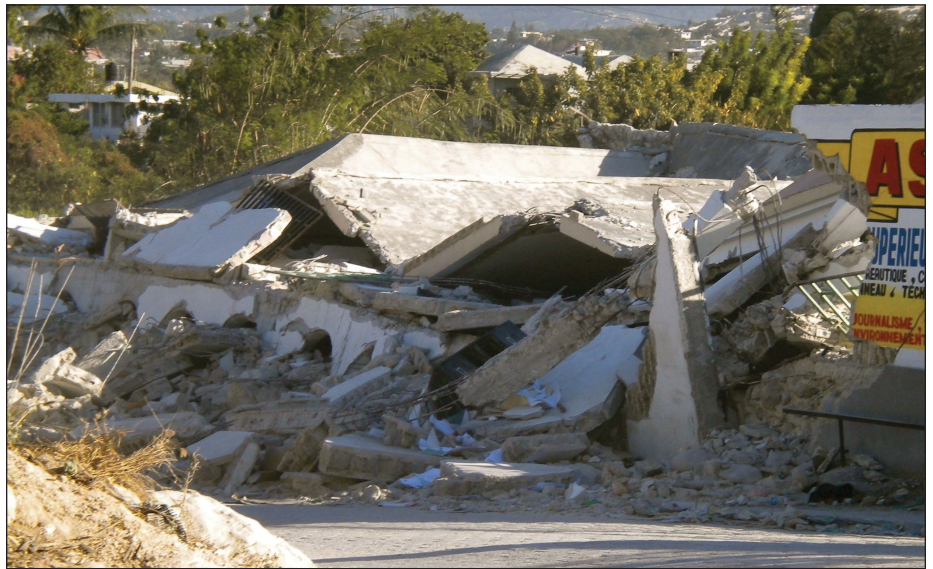
Fig. 1. A collapsed school in Port-au-Prince, Haiti. Photographs were graciously provided by a team of scientists currently in Haiti. More photos and other information can be found at http://haititips.wordpress.com/ . Photo by Andy Freed.
